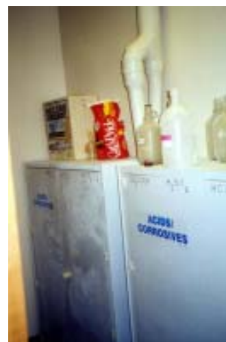
Inadequately vented chemical storage
