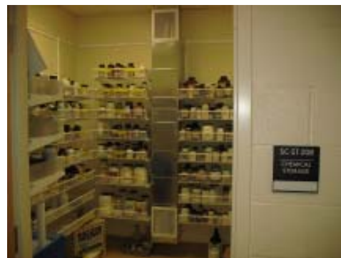
Chemical storage with high and low vents
