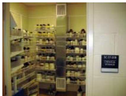
Bi-level ventilation for chemical storage
