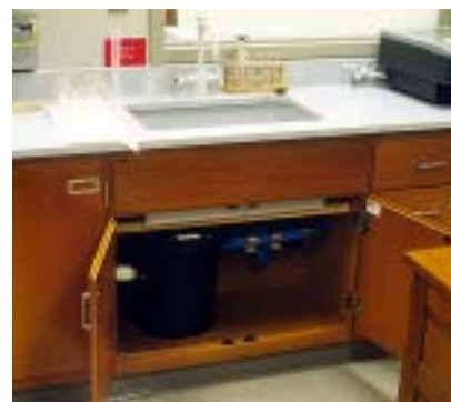
Acid neutralization tank beneath sink
