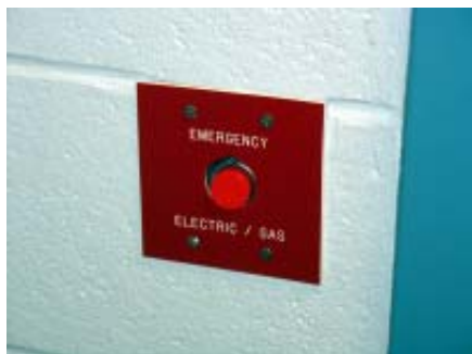
Gas and electric emergency shut-off
