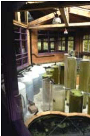
Biological sewage treatment
