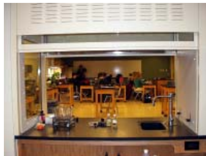
Fume hood between lab and prep room
