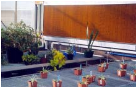
Evaporative cooler on wall
